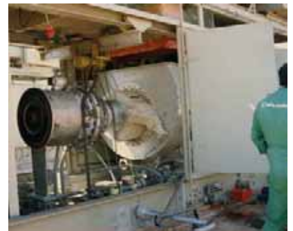
C40 engine under commissioning
